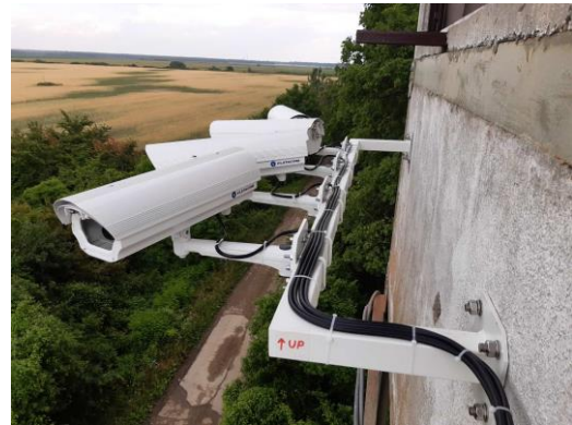
Figure 14. Cameras installed on the watchtower
