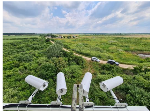
Figure 15. View from watchtower with installed cameras
