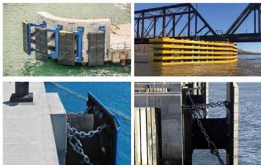
Figure 2. Examples of infrastructure protection systems in a maritime environment
