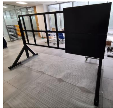
Figure 10. Assembling of monitors for 2x3 video wall
