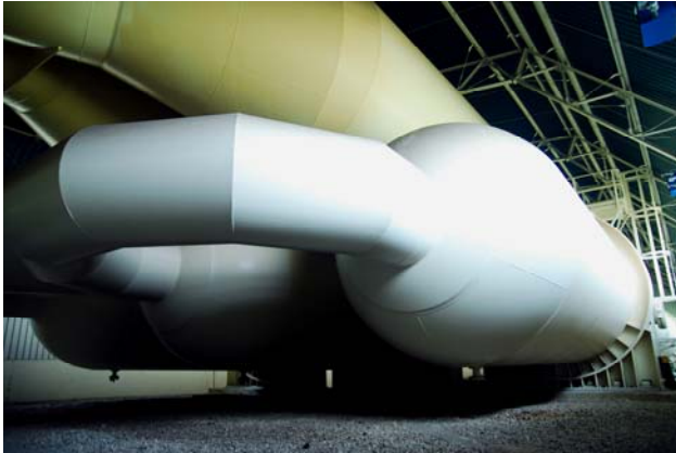
Figure 1. Pressurized air storage tanks of the VTI T-38 wind tunnel
