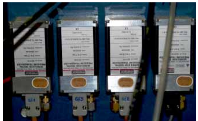
Figure 13. The new pressure transducers installed in the T-38 wind tunnel hall
