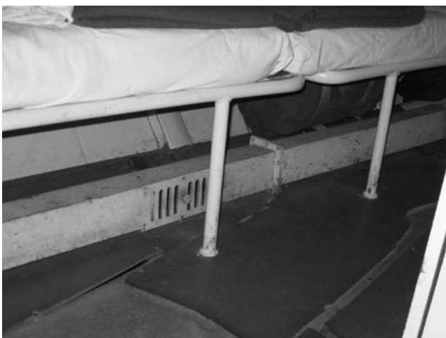
Figure 3. Part of the room heating system - Duct with outlet opening in the sailor cabin
