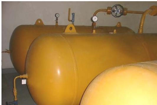
Figure 7. Air storage tanks
