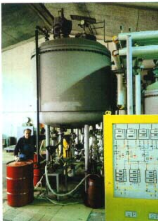
Figure 2. Plant with automatic control for preparing raw materials
